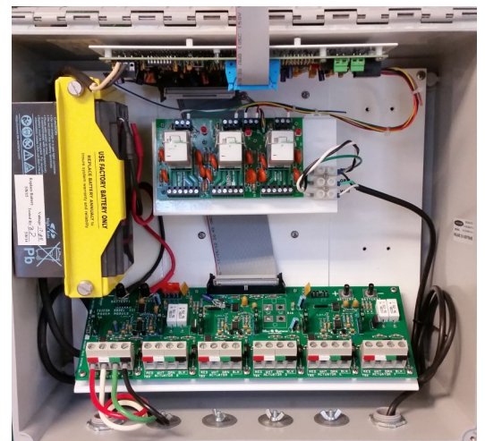
Relay Interface Module Installed
